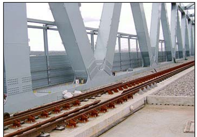
Rheda 2000 Track and turnouts were constructed on viaducts and on steel bridges with special arrangements
